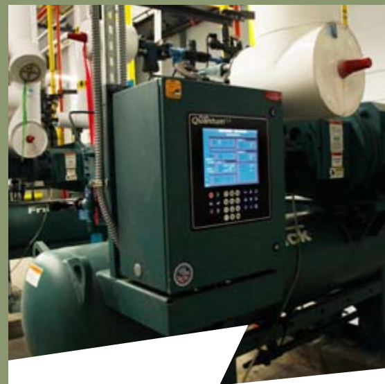
Americold's compressor with control panel.
