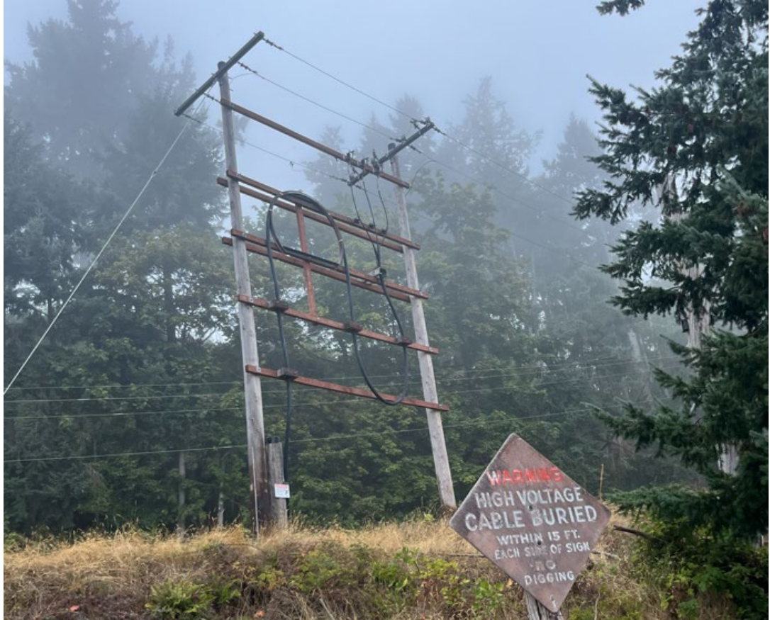
Figure 3. Submarine Cable Riser Structure
