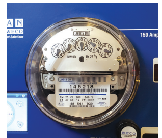
Existing Legacy Electromechanical Meter
