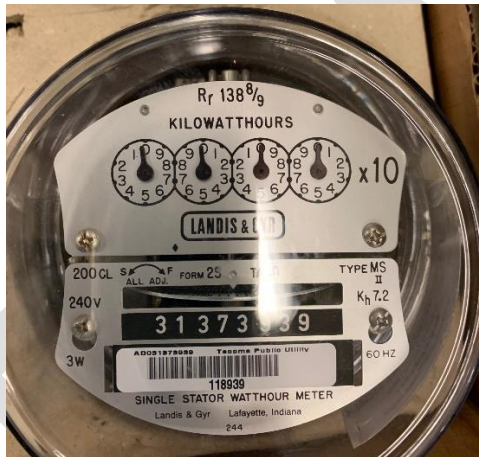
Legacy Electromechanical Meter
