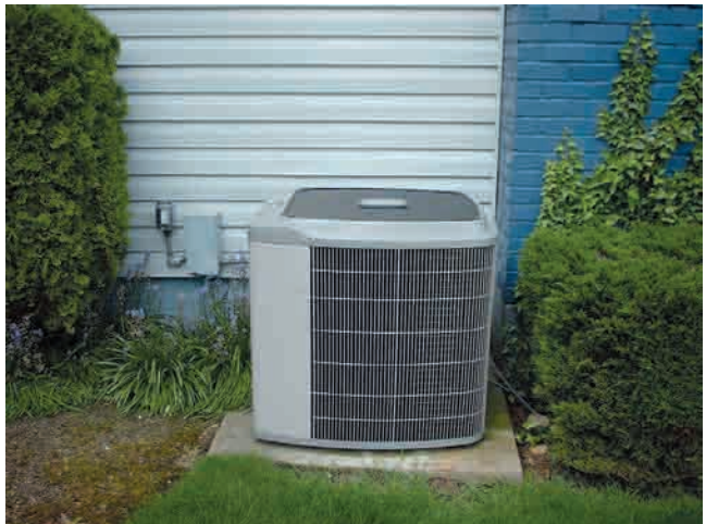
A typical heat pump sits at the back of a house.
